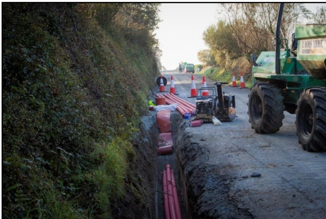
Figure 4-18 Typical ducting installation works for a grid connection cable trench on public road
