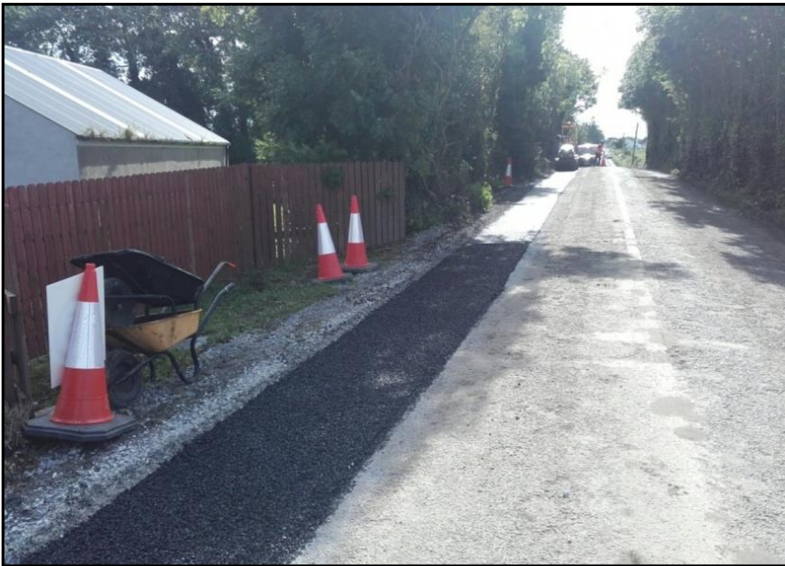
Figure 4-19 Typical permanent reinstatement works for a grid connection cable trench on public road
